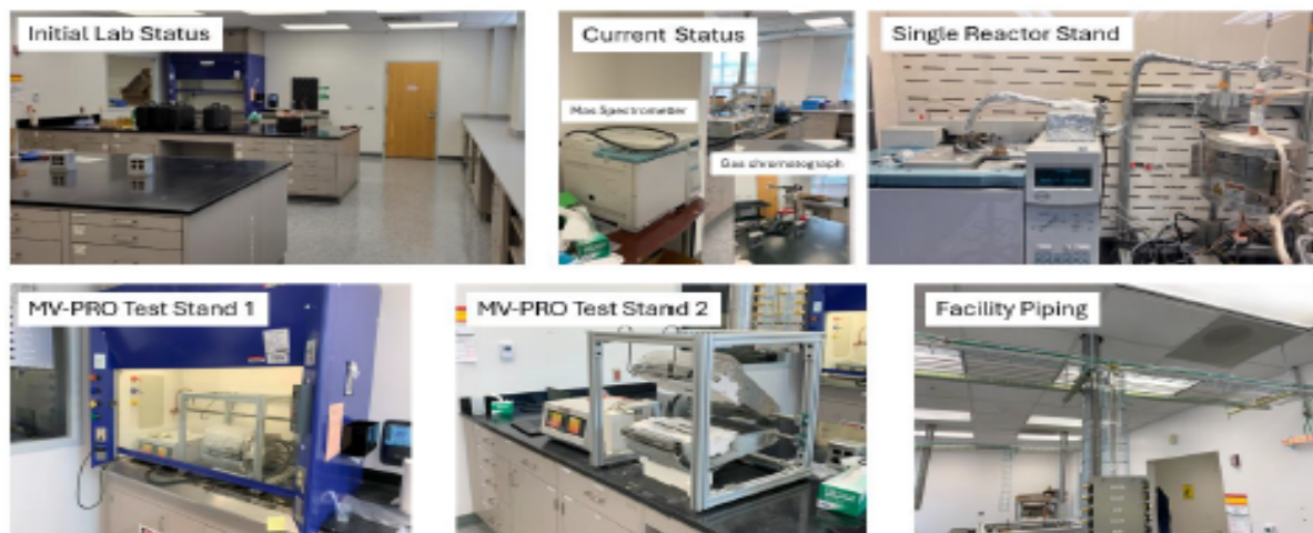
Facility progress status showing multiple commissioned test stands and finalized facility upgrades (gas, electrical, ventilation).
